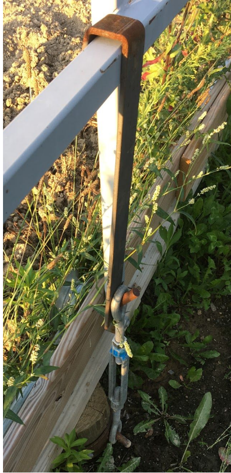
Figure 3: High tunnel anchoring system. Flat steel belt and collar were welded and bent to fit their respective components.
